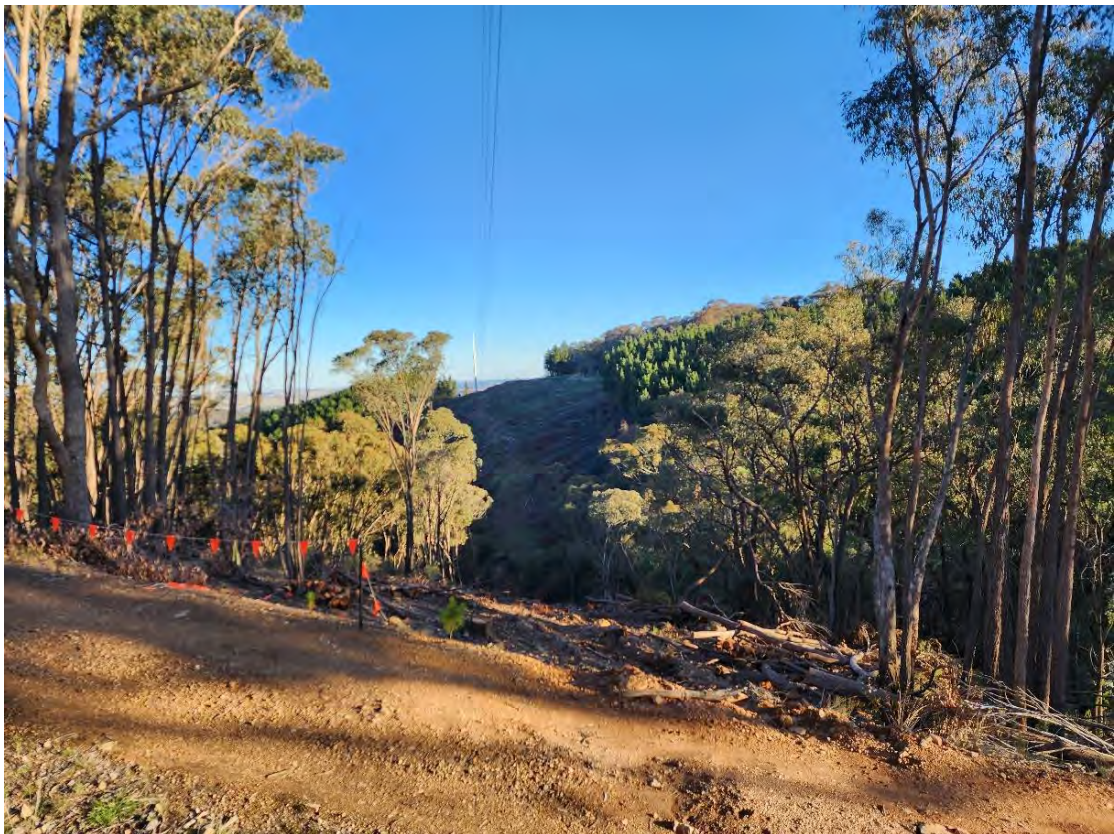
Photos: Construction. Top: Wind turbine pad, laydown area and internal access. Bottom: Reduced width clearing through native vegetation along transmission easement.
