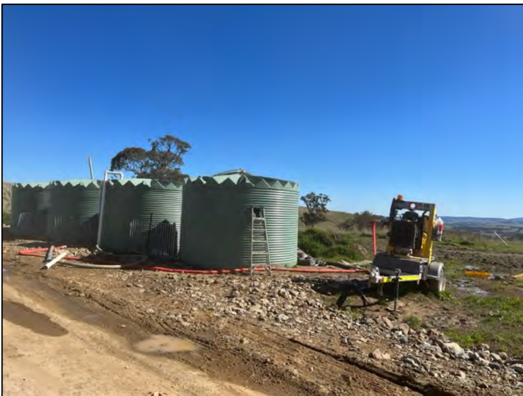
Plate 4: View of fire-fighting water tanks and associated fittings/pump on the Project site.
