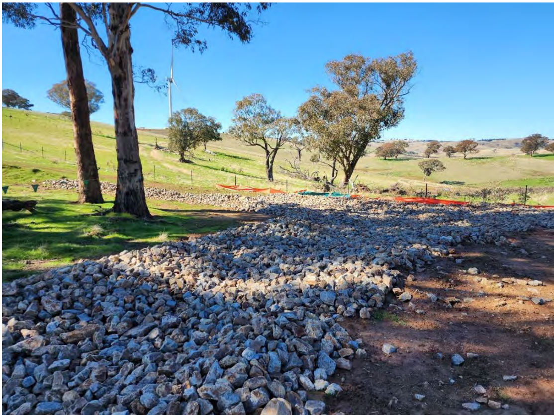
Photos: Erosion and sedimentation control. Top: soil stockpile with sediment control at the base. Bottom: Rubble slowing overland water flow.
