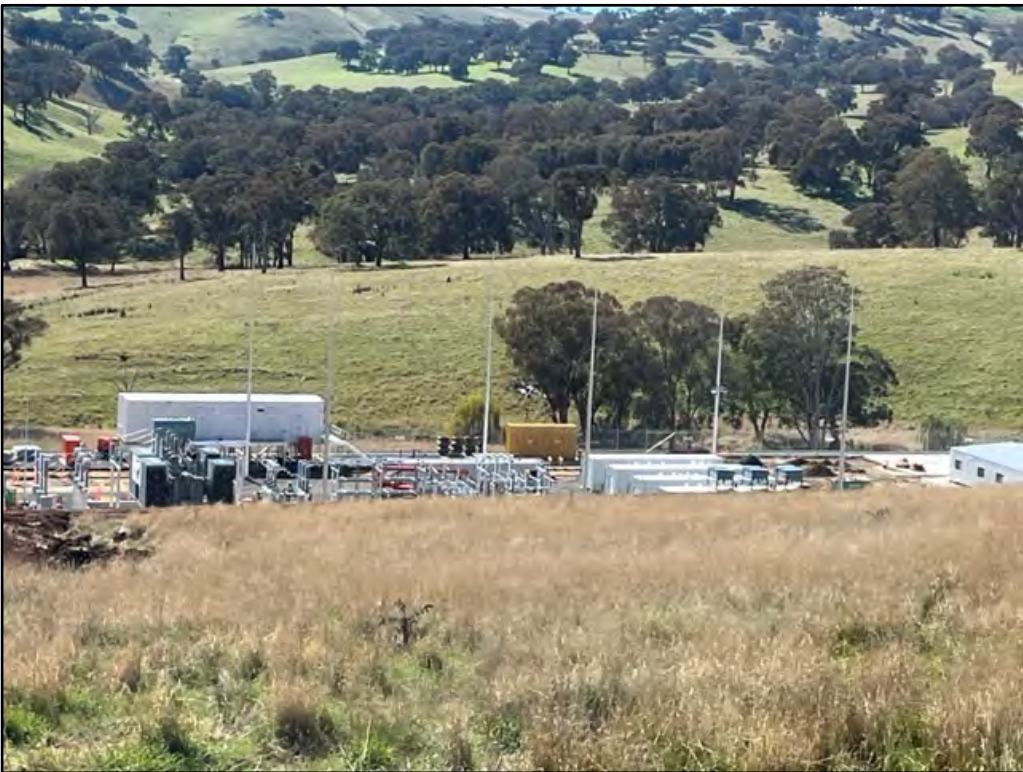
Plate 8: View of electrical substation works. Building colours were noted to be of low-reflectivity and off-white colour.
