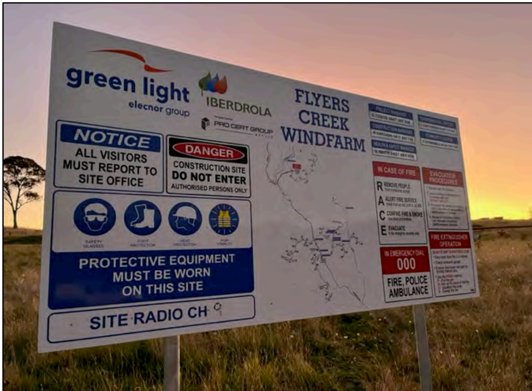
Plate 1: View of signage at the main Flyers Creek Wind Farm construction compound and office showing key project information including contact details.
