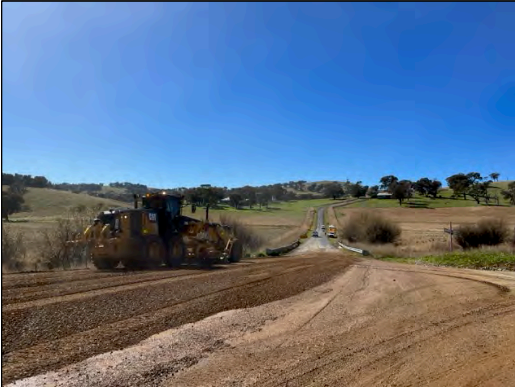
Plate 3: View of road repair/rectification works on roadways adjoining the Project site as observed on 10 May 2023. Works were conducted in consultation with Blayney Shire Council with funding contributions from Flyers Creek Wind Farm.
