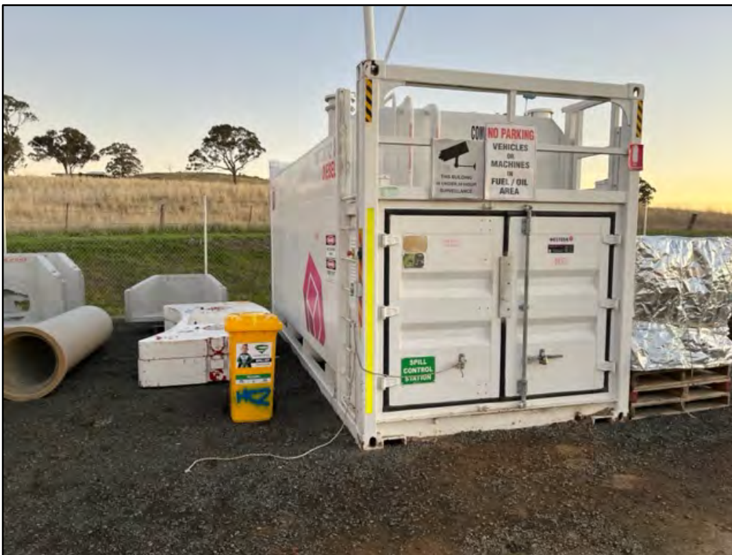
Plate 12: View of the diesel storage and fuelling area within the main site compound. An appropriately stocked spill kit was present at this location. Bunding at the fill point is suggested to minimise risk of spills impacting soils.
